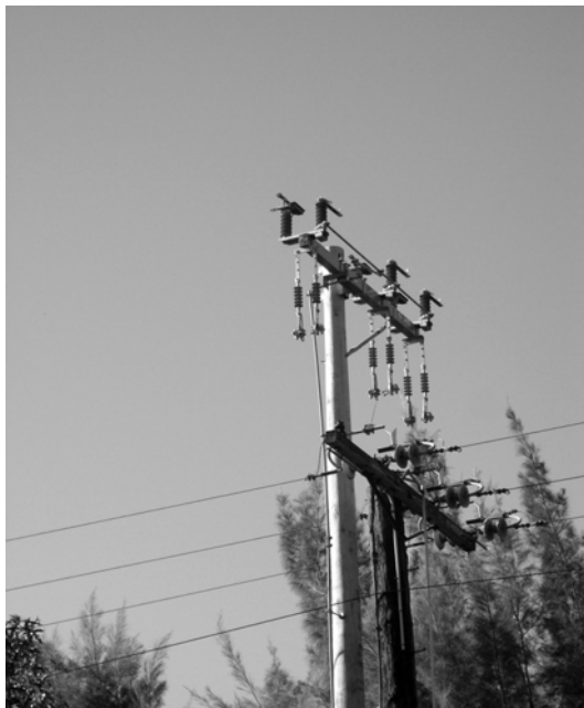
SMUD power poles are being replaced along Moddison Avenue next to the railroad levee.
